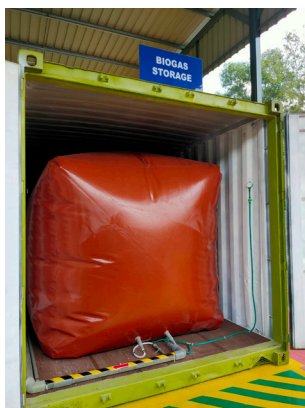
Biogas that had been produced is kept in this 20m 3 capacity storage bag.
