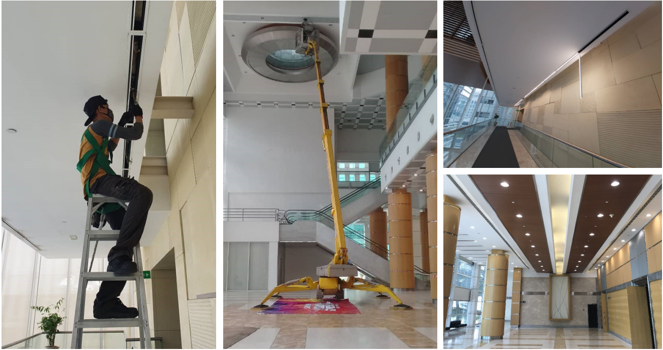
LED lights and motion sensors are fitted at office block corridors and hall's lobby area.
