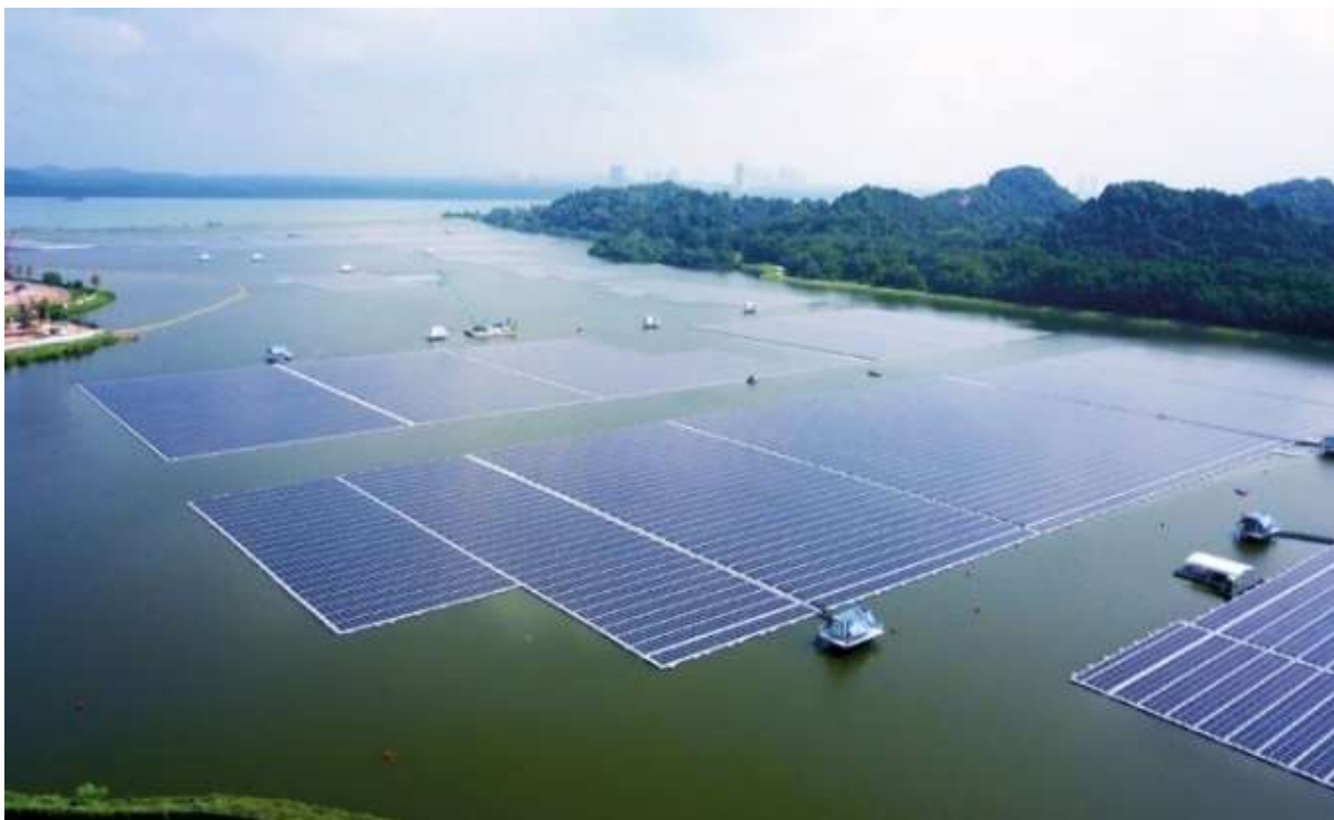
Photo 2: Example of floating solar farm in Singapore (Sembcorp Tengeh Floating Solar Farm) Source: https://www.futurarc.com
