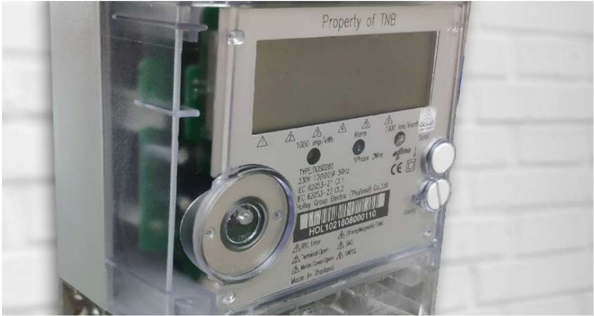
Photo 6: Smart meter Source: https://www.mytnb.com.my/smart-meter
