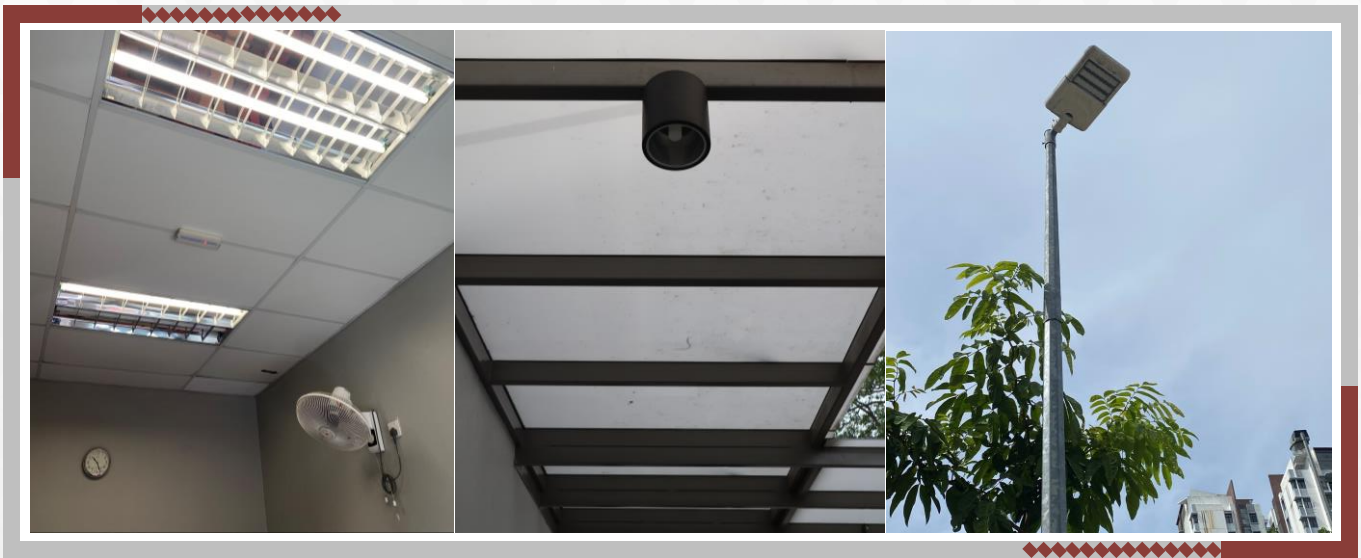
Most of the lights used are energy-efficient types, namely LED and T8 lamps. Suggestions for improvement can be made by installing lux sensors/motion sensors to optimize energy usage.
